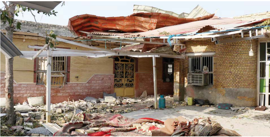
Rubble lies around a damaged house following a reported attack near a wedding gathering in Kuhistik, Sirik, Iran.
